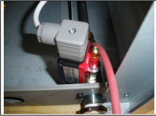
Fig 7.2.2 - Gas Inlet Pressure Test Point
