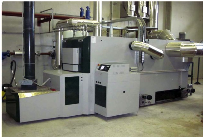
Typical plant room with 800 kW BioFire biomass boiler and vertical fuel feed.
