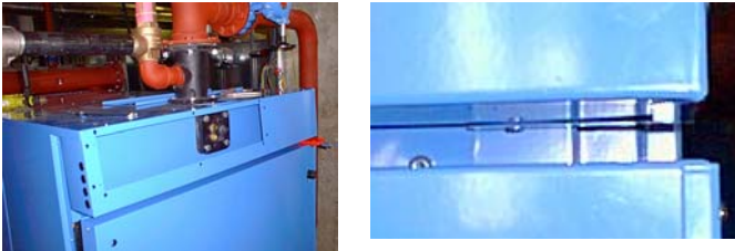
Picture 12: Control Box
