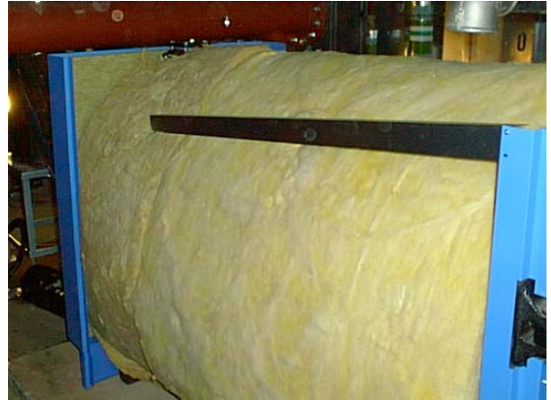
Picture 5: Boiler Body Insulation
