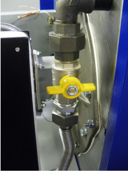
Figure 8.1.1 - Gas Isolating Valve
