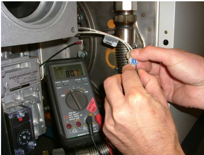
Figure 7.2.3 - Hot Surface Igniter Check (196/ 254 shown with air filter removed)
