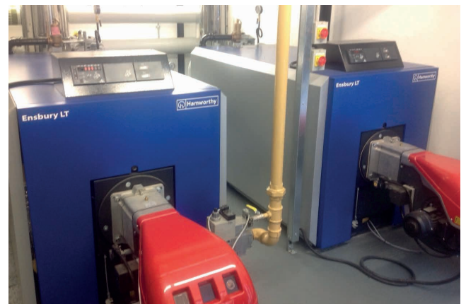
Ensbury pressure jet boiler
