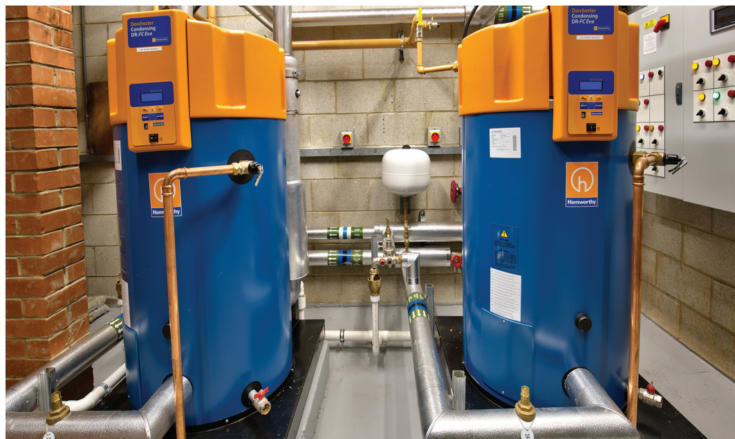
Two DR-FC Evo water heaters installed at Abbey Hill Academy.
