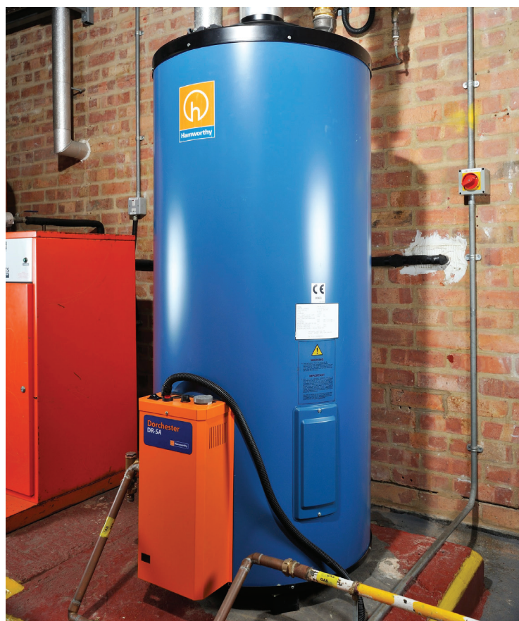
Dorchester DR-SA automatic ignition direct-fired water heater in a plant room
